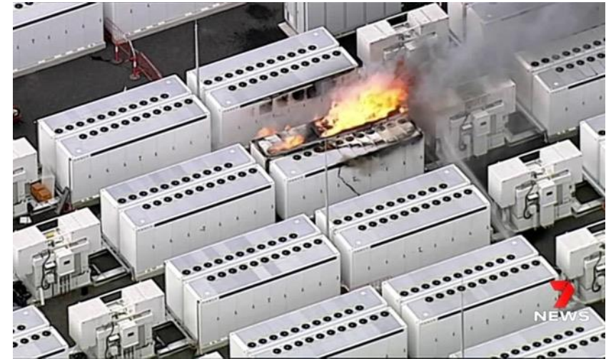
Stationary lithium battery fire Victoria
